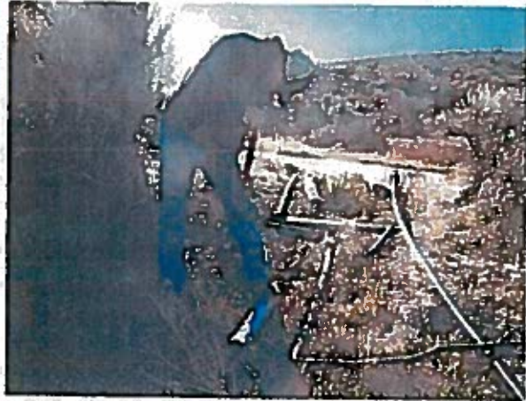
Installing a pipe in order to measure surface outflow from R04233 pond.
