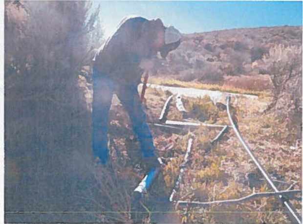
Installing a pipe in order to measure surface outflow from R04233 pond.
