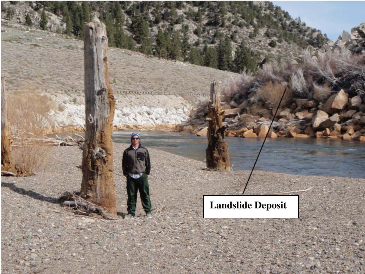
Figure 2.1-106. Landslide deposit and highway.
