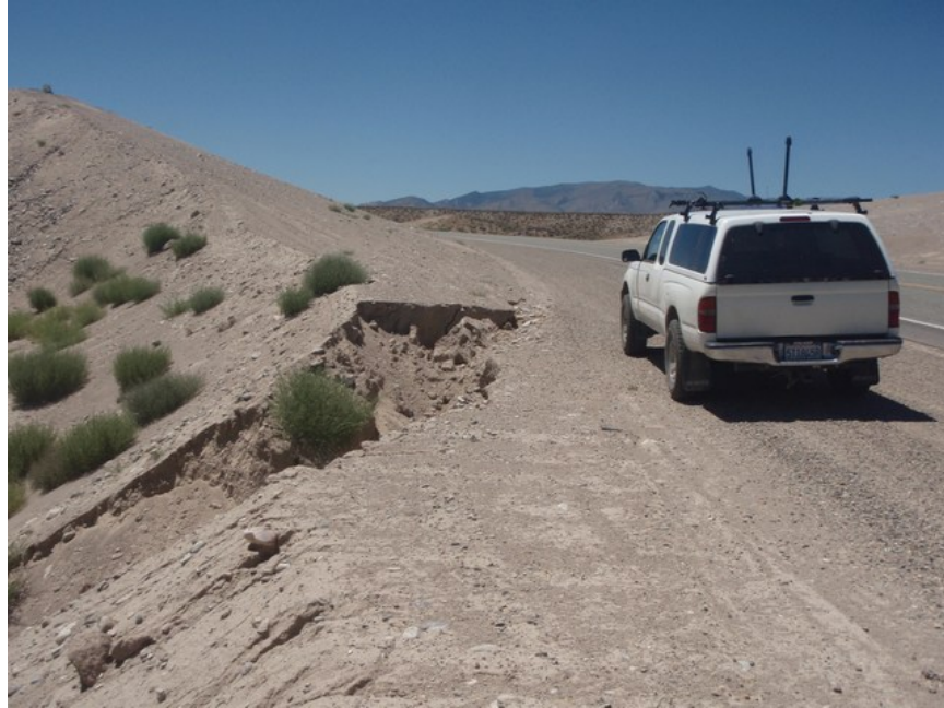
Figure 2.1-124. Large gully erosion off of highway fill slope near Wilson Canyon. The cutslope has just been regraded and no BMP's were evident.
