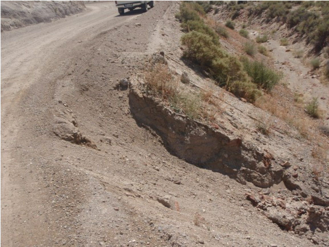
Figure 2.1-126. Side-cast berm has collapsed into the drainage.
