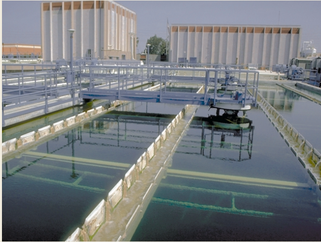
Water Factory 21 treatment facility. (Photograph courtesy of Orange County Water District.)
