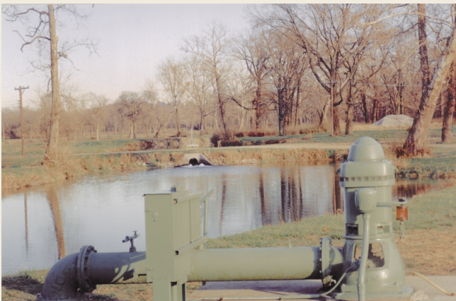
High-capacity turbine pump installed on a municipal well at Rohrsers Island. Recharge lagoon in background. (Photograph by Brent Means, U.S. Geological Survey.)
