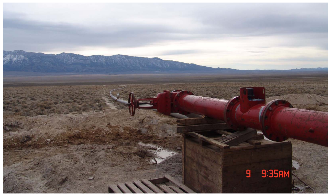
Figure A-4 Discharge Piping, Facing East from Well Site 184W105
