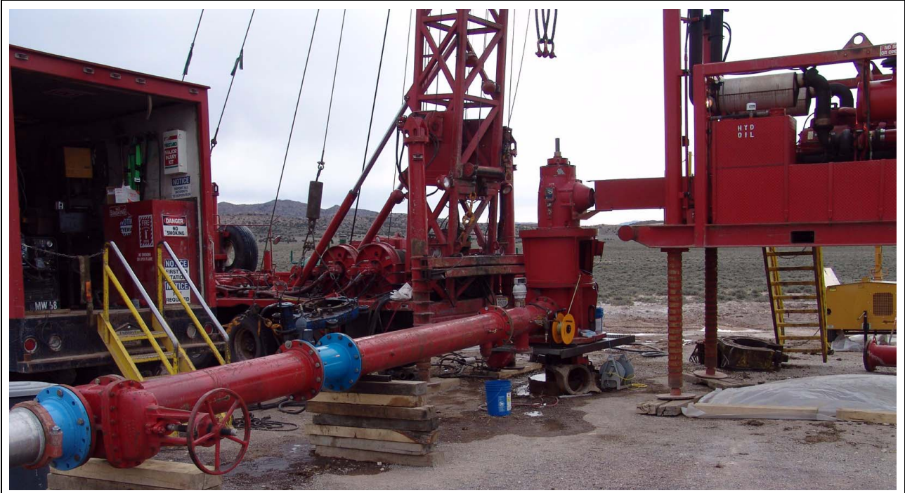
Figure A-2 184W101 Test Wellhead Equipment and Site Setup
