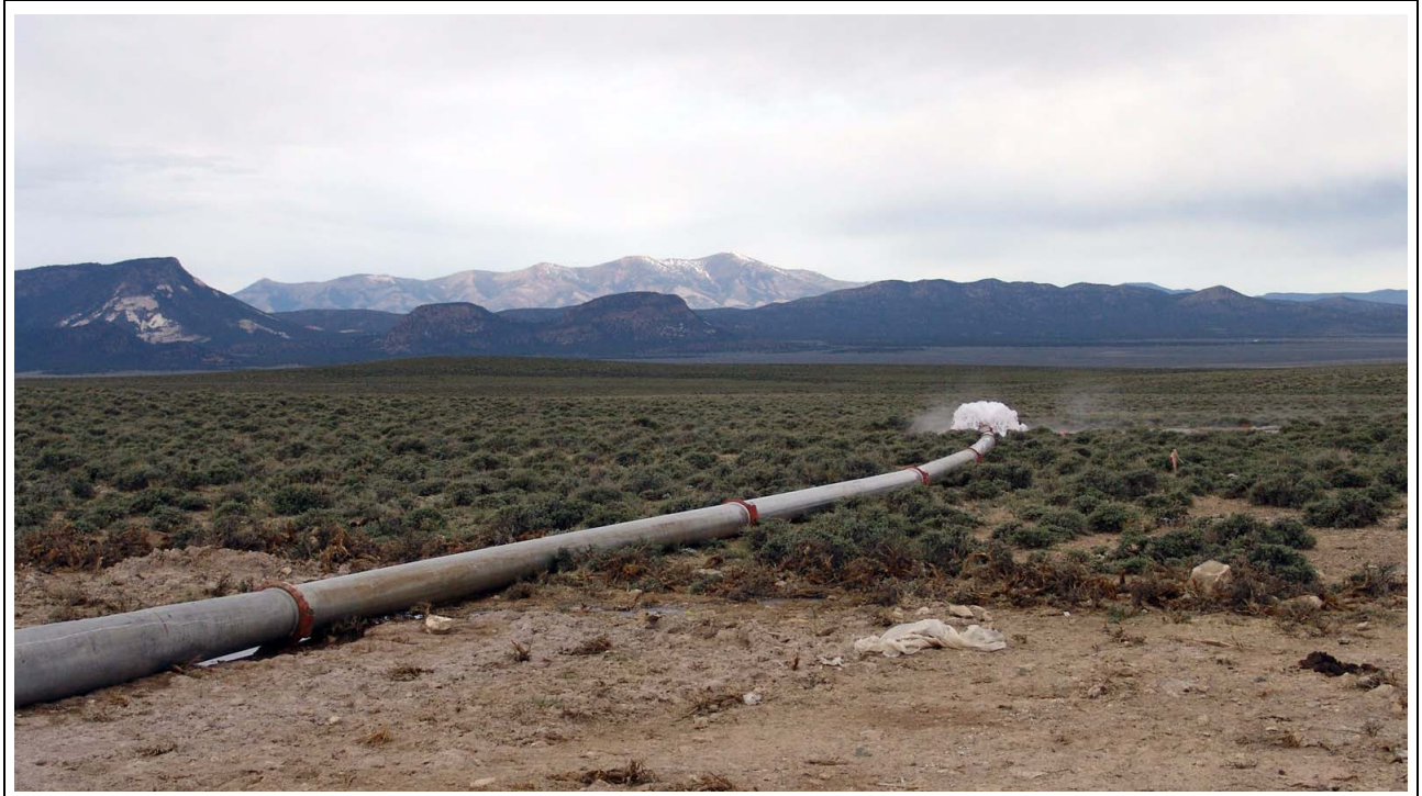
Figure A-4 184W101 Discharge Line
