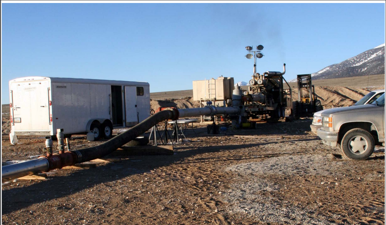
Figure A-1 Test Well SPR7007X Wellhead Hydraulic Testing Equipment and Discharge Line
