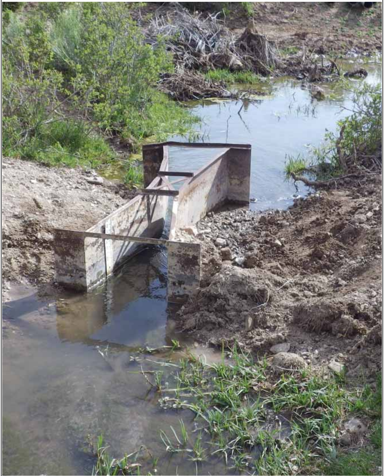
Figure E-7 Parker Station Flume, May 2014
