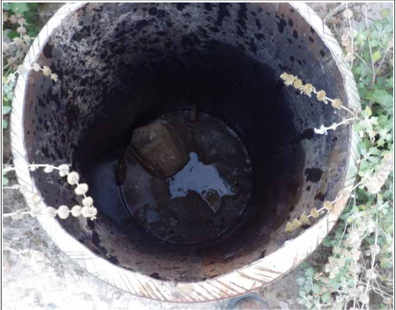
Figure E-10 Lewis Well Spring Collector Line Access Discharge, October 2014
