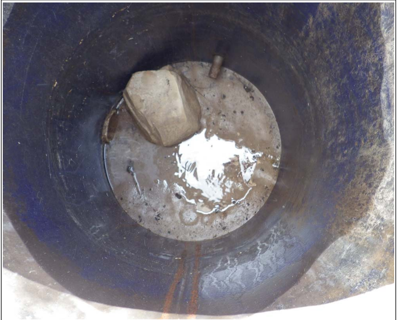
Figure E-10 Lewis Well Spring Collector Line Access Discharge, October 2015
