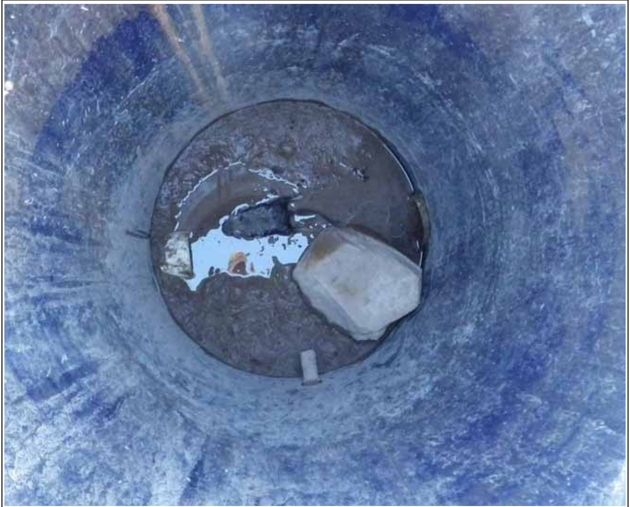
Figure E-10 Lewis Well Spring Collector Line Access Discharge, October 2016
