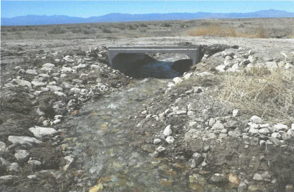
FIGURE 3. New box culvert that replaced the old “40ft culvert” on Sunnyside Creek. This new culvert allows up- and downstream movement of native fish, thus increasing available habitat.
