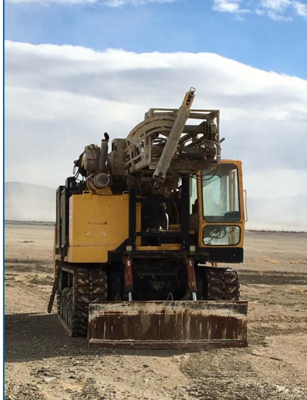
Caterpillar tracks and a dozer blade help this rig operate in the desert playa.
