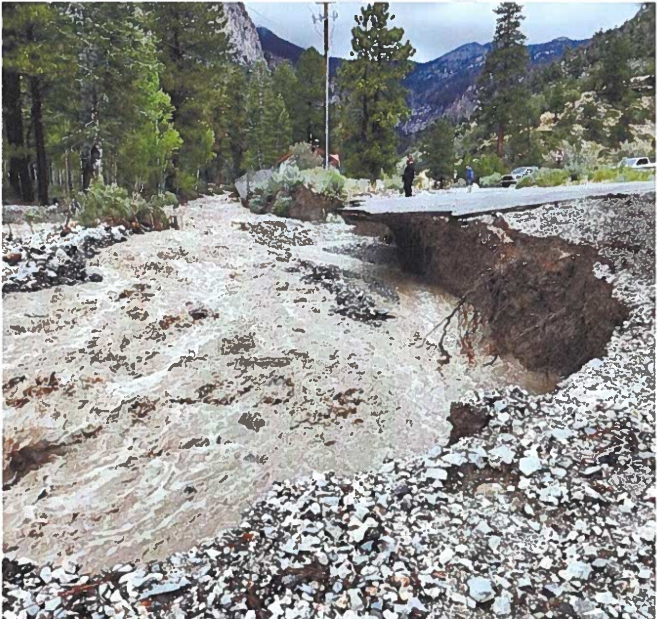
Image: Damage from Tropical Storm Hilary, August 2023
